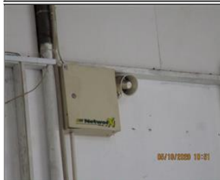
Photo of fire safety equipment Fire alarm.JPG
