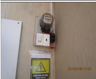
Photo of non-conformity Finding 7.13_No safety cover for electrical panel.JPG
