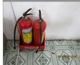
Photo of fire safety equipment Fire extinguishers.JPG
