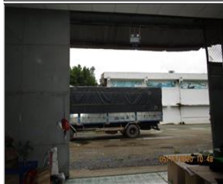
Photo of non-conformity Finding 7.15_Emergency exit at production workshop as sliding door.JPG
