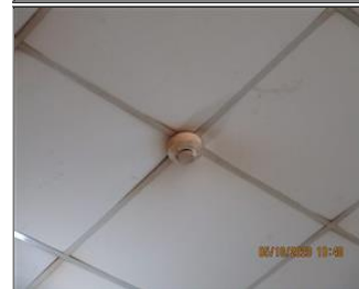
Photo of fire safety equipment Smoke detector.JPG
