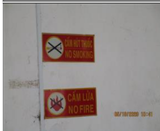
Photo of fire safety equipment No smoking warning sign.JPG
